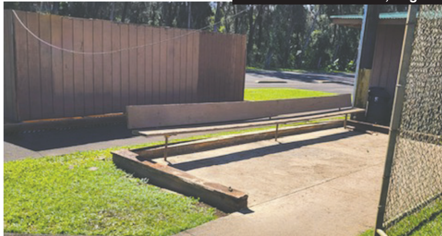
Photos by Shirley Garcia Nakamura A photo timeline of the dismantling of the old dugout and construction of the new one at Kamehameha Park by Kohala's kupuna softball team Local Boyz.
